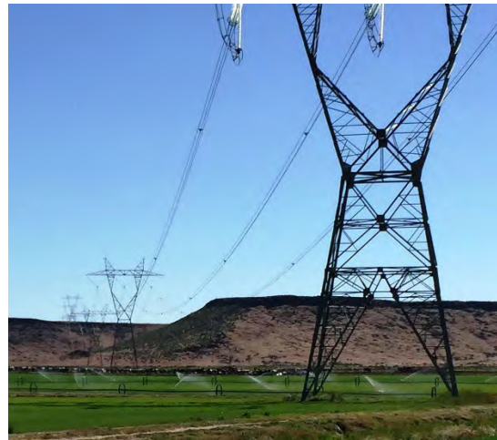
500-kilovolt (kV) transmission line near Melba, Idaho
