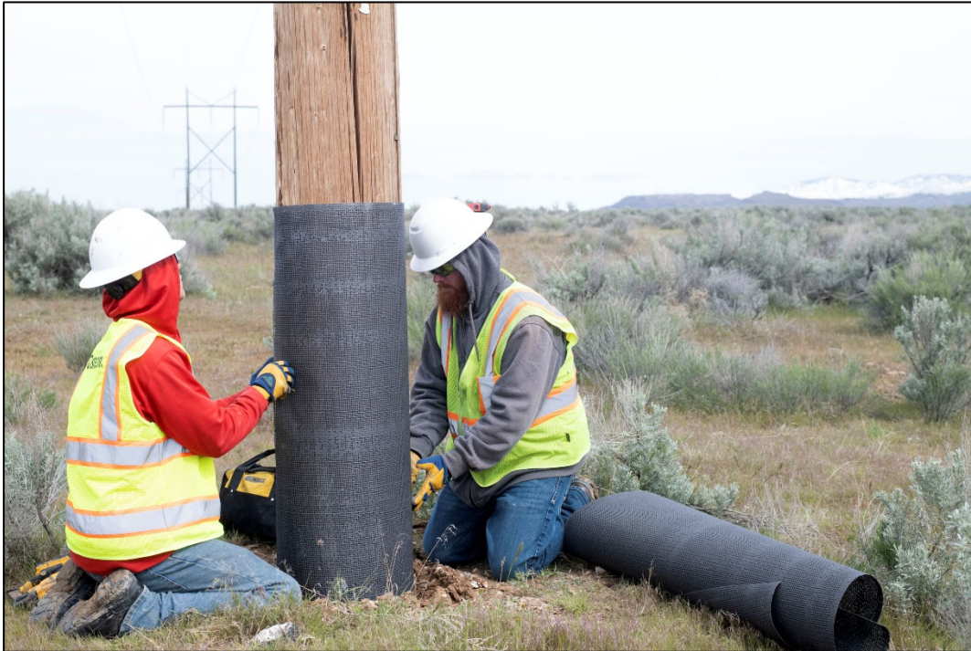
Figure 1. Idaho Power Field Personnel Apply a Fire-Resistant Mesh Wrap to a Transmission Pole (2022)
