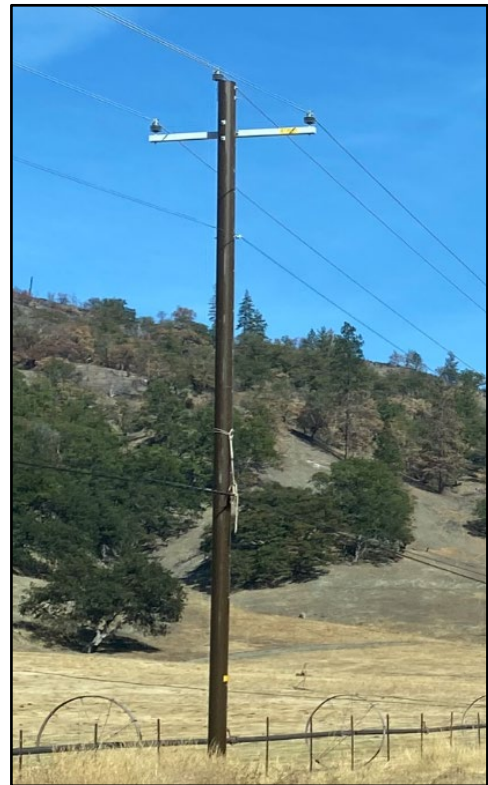
Figure 19: Distribution Fiberglass Poles
