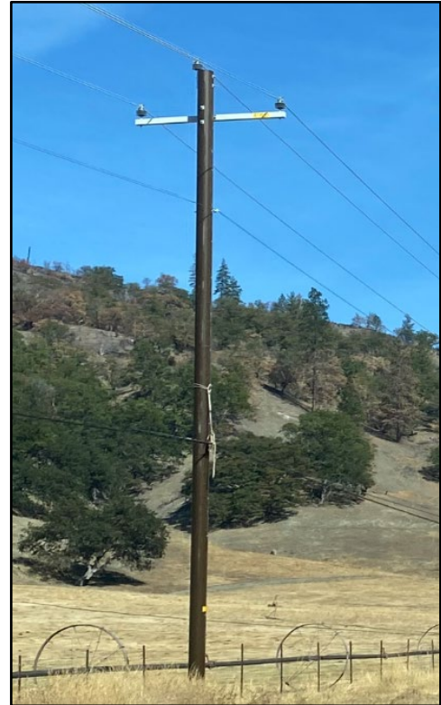
Figure 19: Distribution Fiberglass Poles
