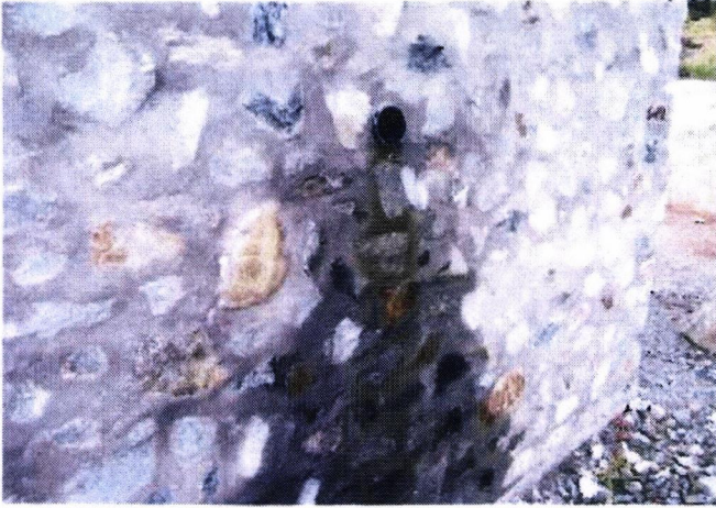
Flow to waste valve leaking
