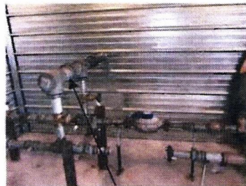
Flow to waste line and flow meter
