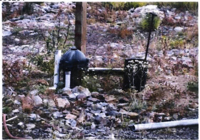
Well #2 - not hooked up
