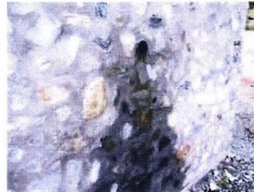
Flow to waste valve leaking
