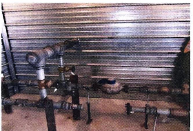
Flow meter and flow to waste line
