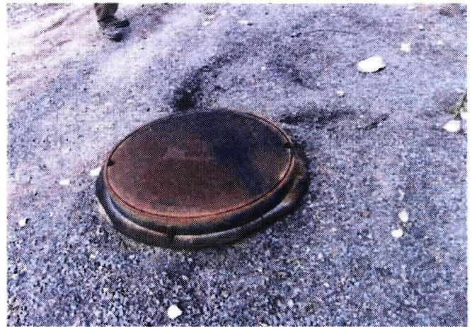
Air relief vault
