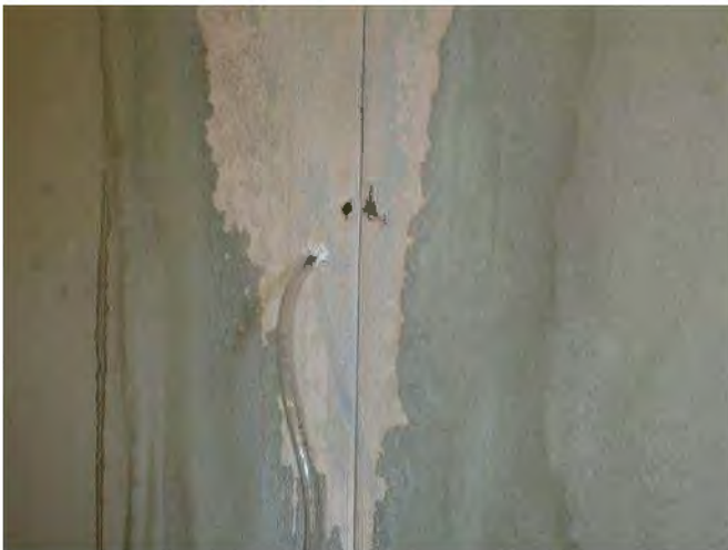
Photograph 13: Interior plastic tube to vent chlorine to outside
