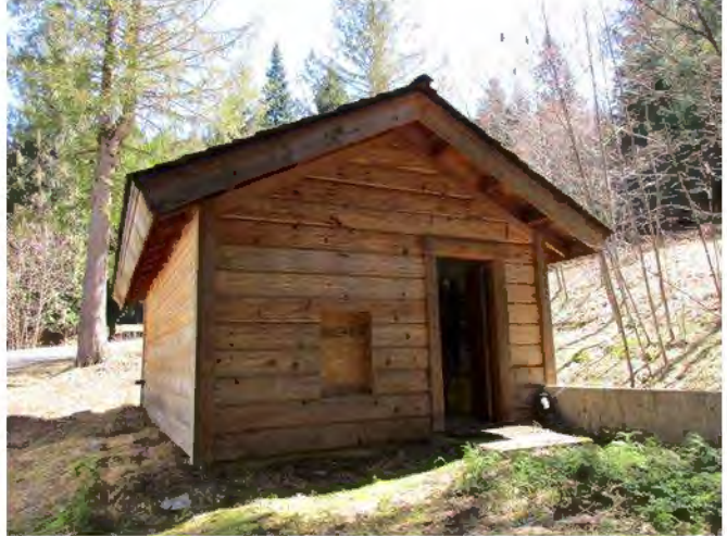
Photograph 40: Booster station 1 (lowest) on south side of hwy 200
