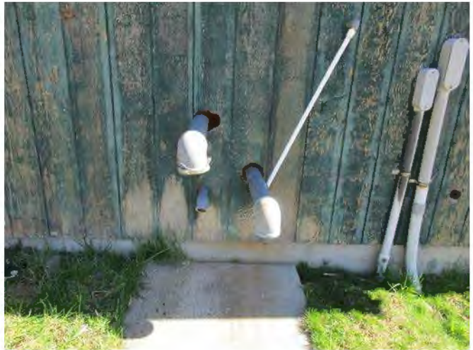
Photograph 20: Concrete slab under well flow to waste
