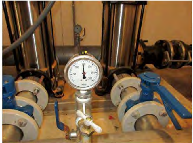
Photograph 54: Pressure guage at BS1, pumps up to Southside Hilltop storage tank
