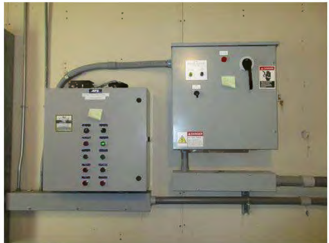
Photograph 14: Electrical components inside pump house
