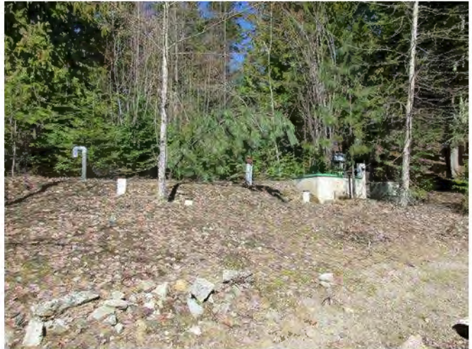
Photograph 22: Mid level underground storage tank (MLST), hatch riser, vents
