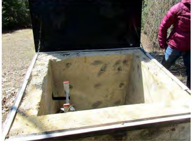
Photograph 36: UST Concrete deterioration around hatch lid area
