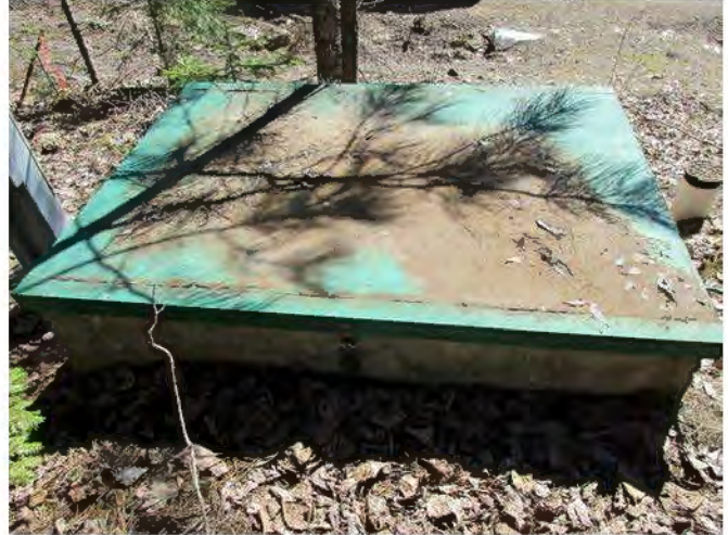
Photograph 26: MLST Steel lid on hatch, locked
