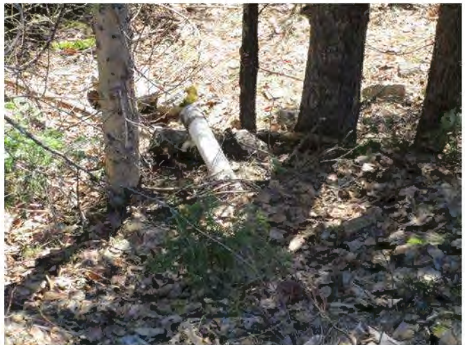
Photograph 24: Flow to waste with screened end cover MLST
