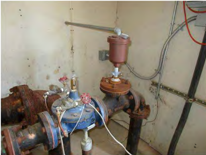
Photograph 9: Pressure relief valve & flow to waste
