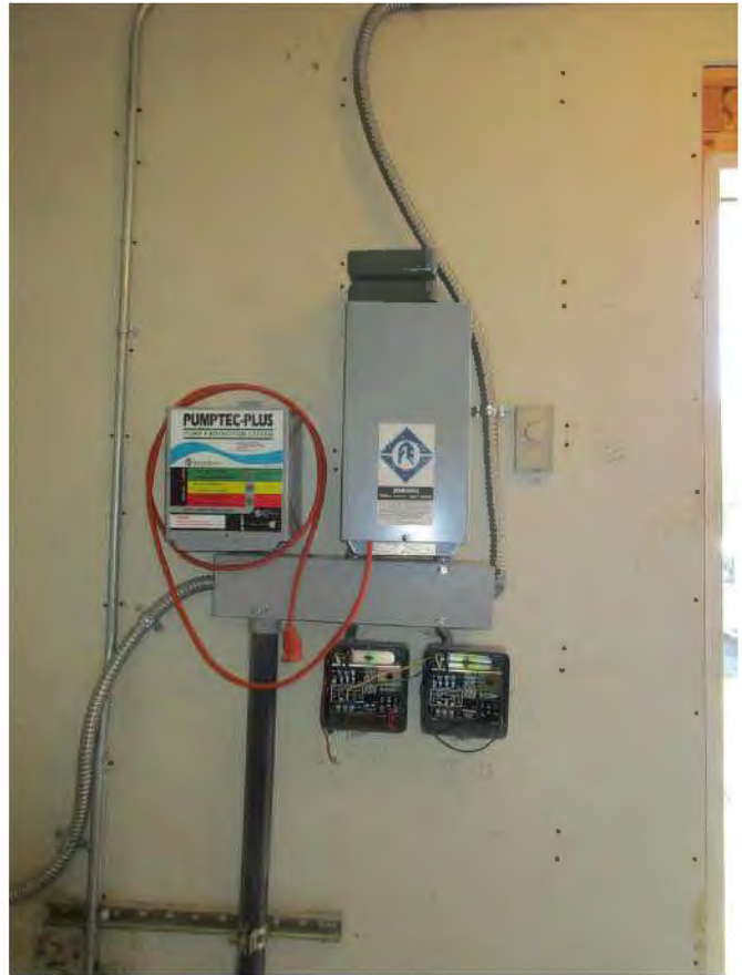
Photograph 8: Pumptec-Plus pump protection system (auto cut off)
