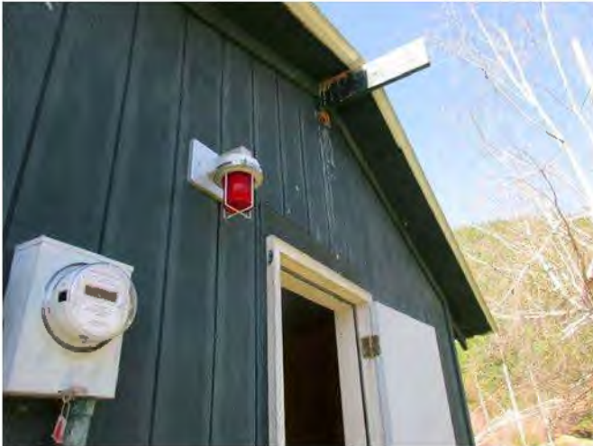
Photograph 21: Pump house entry door and alarm light
