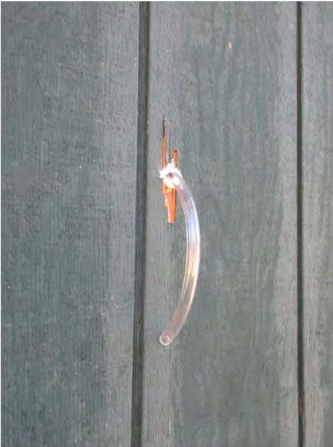
Photograph 17: Exterior view of plastic chlorine vent to outside
