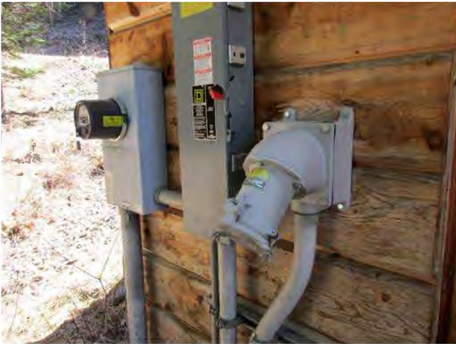
Photograph 57: Ready connection for portable generator to connect on outside wall BS2
