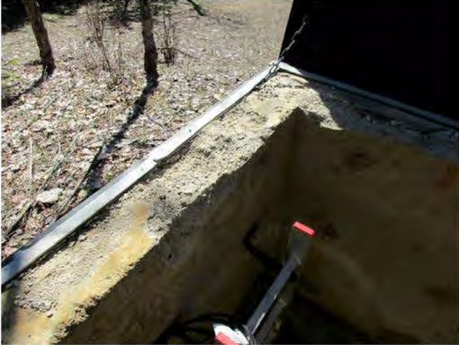
Photograph 35: UST Deteriorating concrete at hatch seal, seal needs to be replaced
