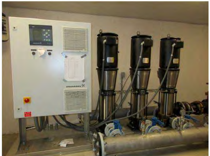
Photograph 46: 20 hp VFD pumps and control panel
