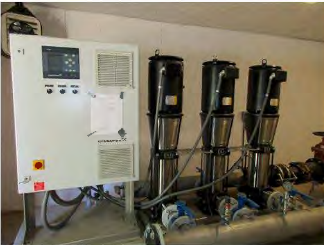
Photograph 59: 20 hp VFD pumps and control panel
