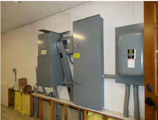
Photograph 45: Electrical panels inside booster station 1
