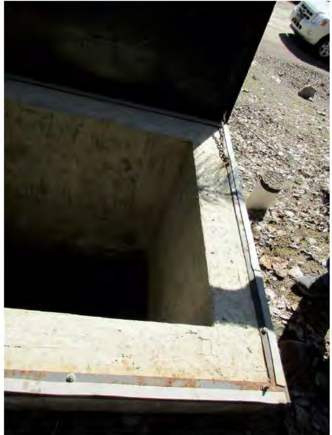
Photograph 28: MLST Hatch seal needs to be replaced
