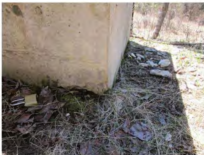
Photograph 33: Concrete deterioration on UST
