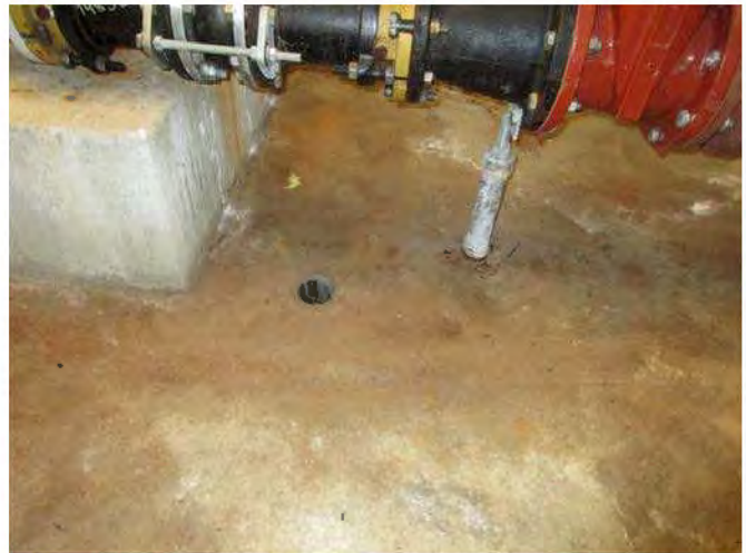
Photograph 50: Floor drain BS1
