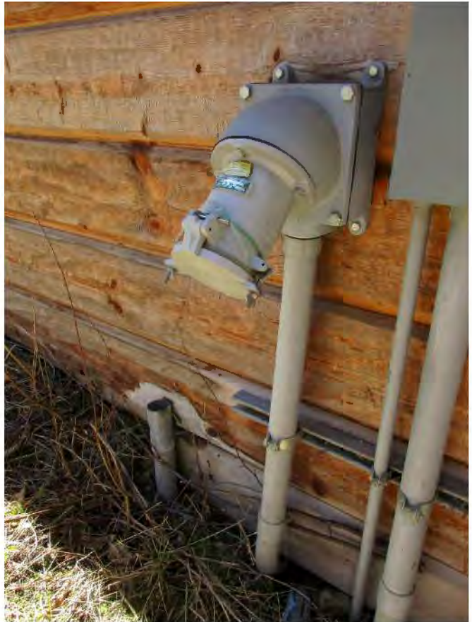
Photograph 42: Ready connection for portable generator to connect
