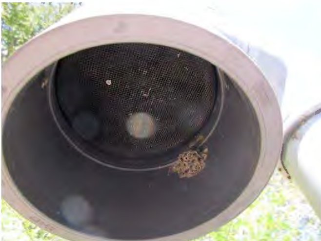
Photograph 23: Screened vents on MLST
