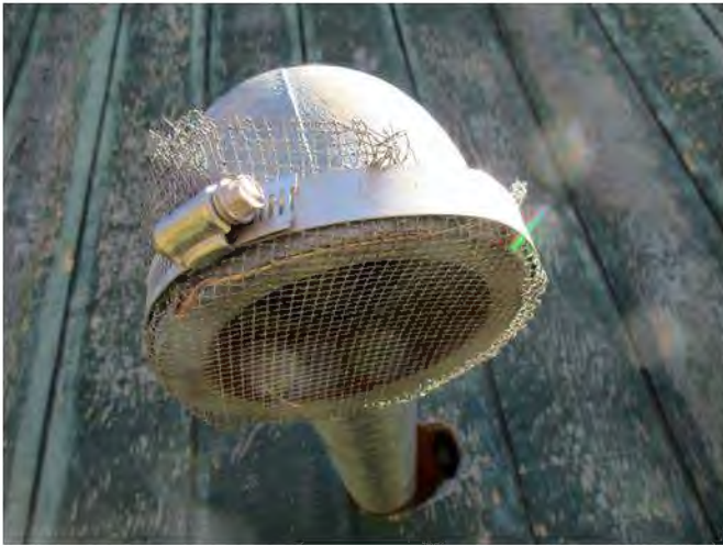
Photograph 19: Screened ends on flow to waste
