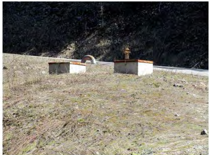
Photograph 56: Vaults at booster station 2 (upper)
