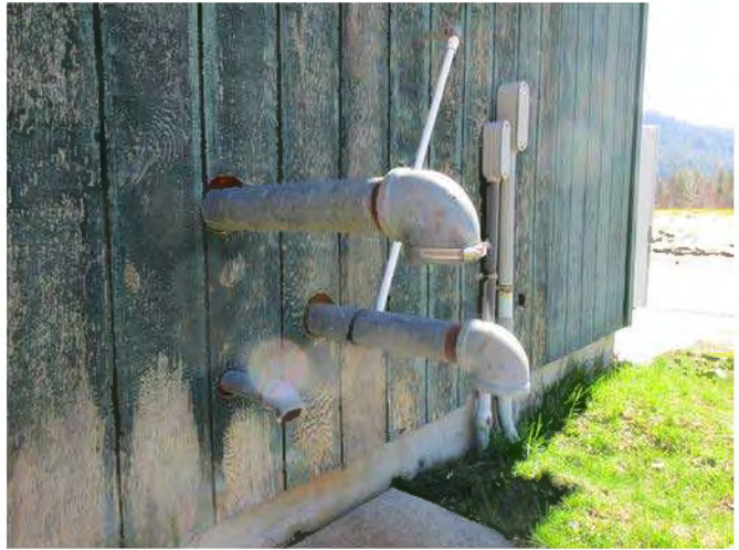
Photograph 18: Well 1 & well 2 flow to waste
