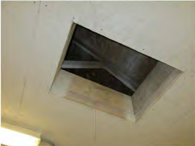
Photograph 53: Open ceiling hatch to improve ventilation
