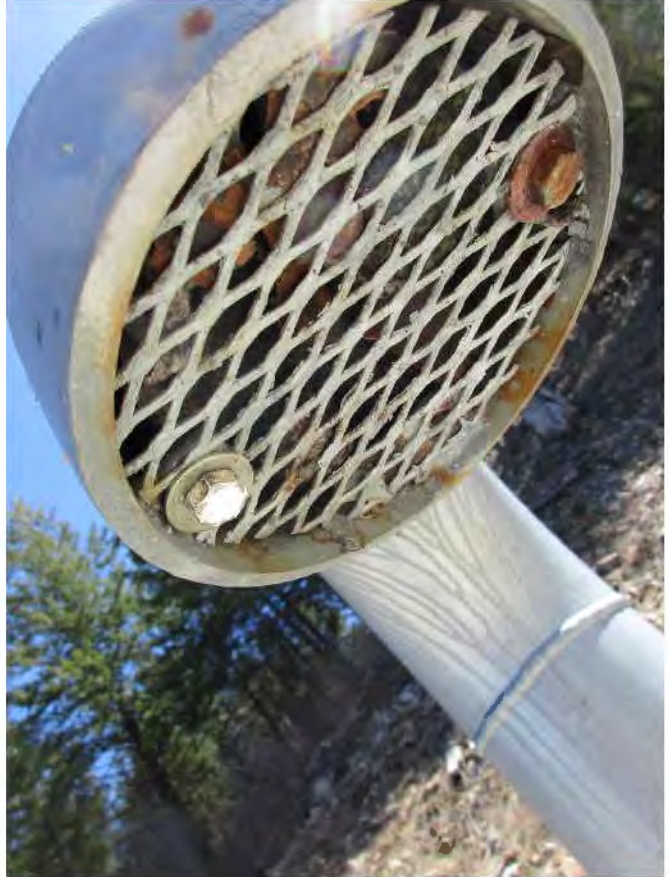
Photograph 64: Screened vents on SHST
