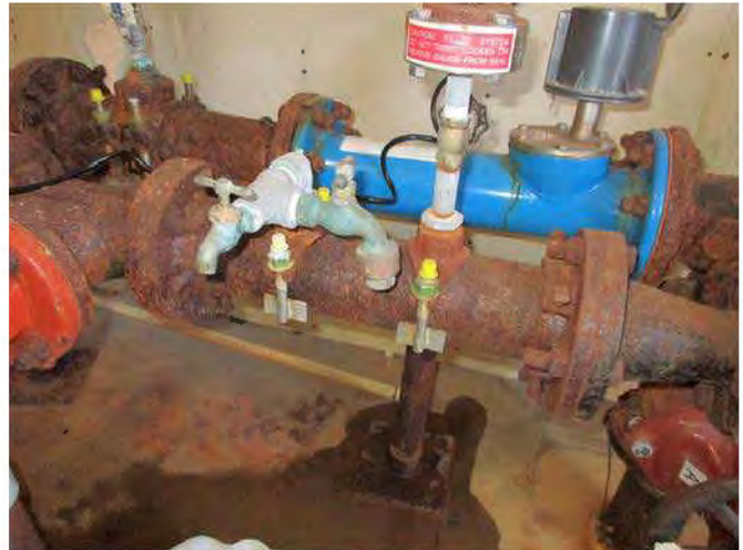
Photograph 10: Sample tap for source sample purposes, also threaded tap with AVB
