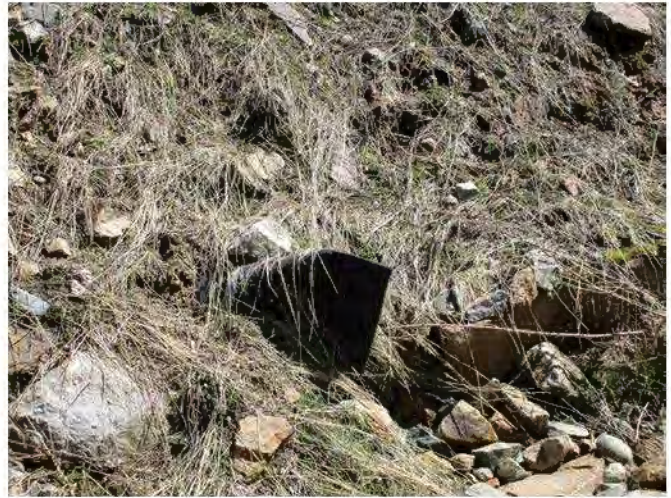
Photograph 70: SHST Flapper valve on overflow/drain
