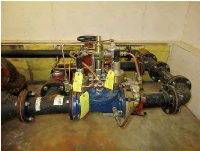
Photograph 49: Valve, backflow and pressure components
