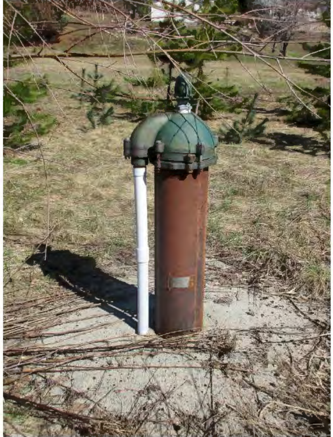
Photograph 4: Well 2 (primary well)
