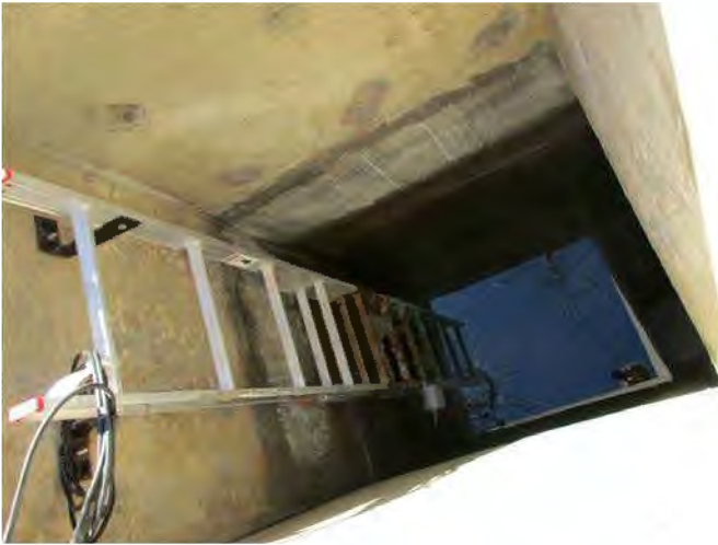
Photograph 37: View into UST, concrete chips on ladder rungs
