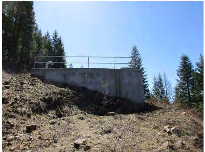
Photograph 62: Side view Southside Hilltop storage tank (SHST) 225K gallons
