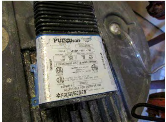
Photograph 12: Pulsatron metering pump for chlorine injection (voluntary)
