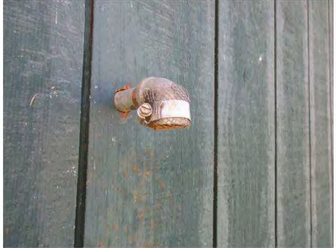
Photograph 16: Pressure relief valve discharge to outside, screened
