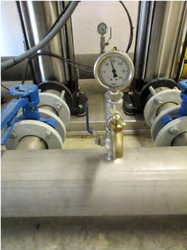
Photograph 61: Pressure guage at BS2
