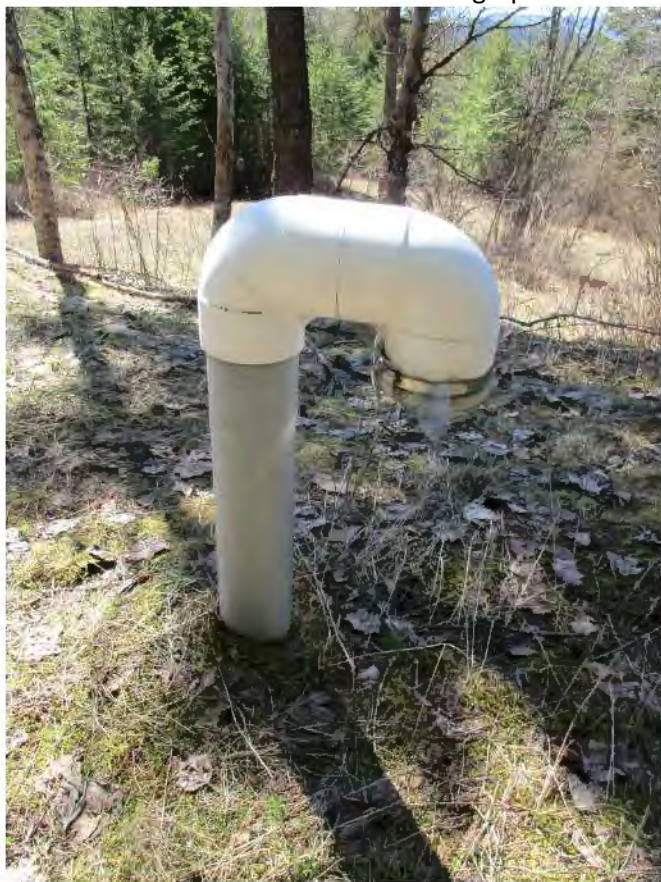
Photograph 31: Screened vent on UST
