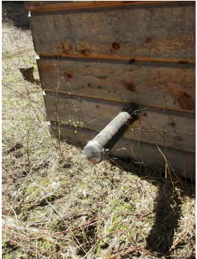
Photograph 58: Screened flow to waste at BS2
