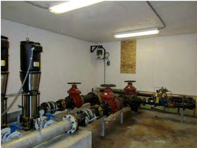
Photograph 47: View of valves, heater, pressure relief valve inside BS1
