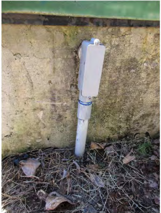
Photograph 38: UST Intact conduit at hatch lid, repaired since previous survey
