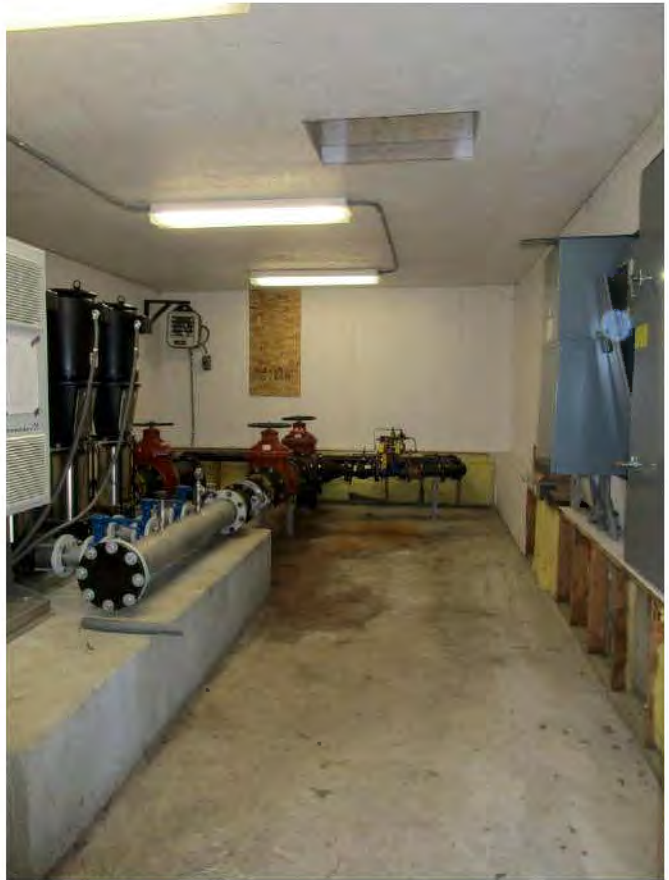
Photograph 44: Inside view of booster station 1 (BS1)
