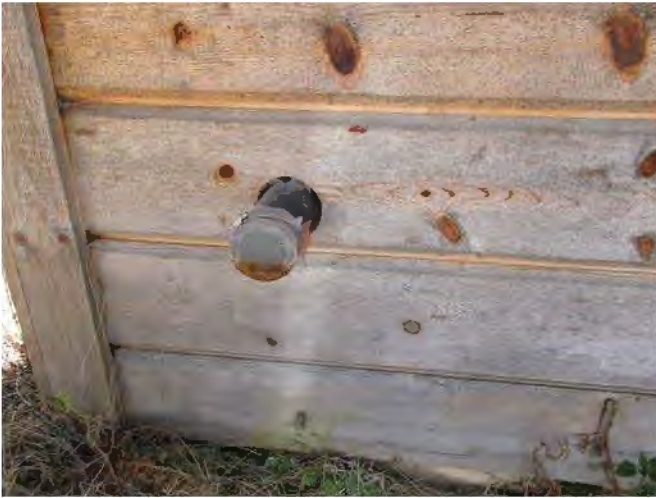
Photograph 41: Flow to waste for VFD pumps
