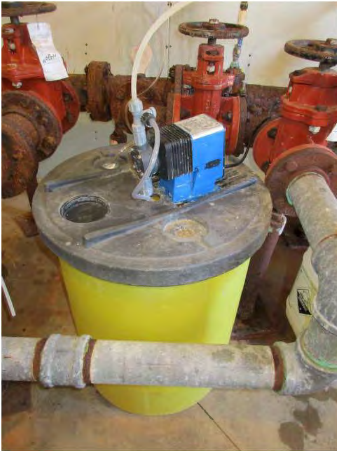
Photograph 11: Chlorination tank with metering pump, vent tube to outside (hole in tank needs to be sealed)
