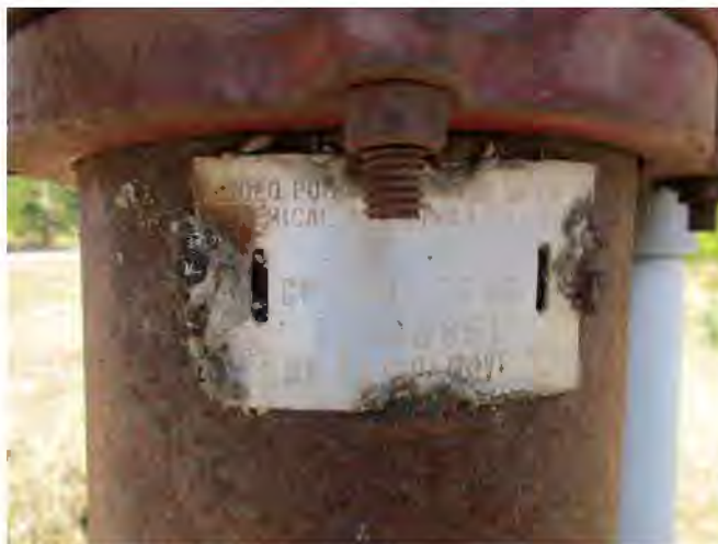
Photograph 2: Well 1 well tag E0005651
