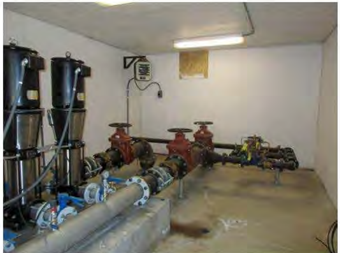
Photograph 60: Inside view of BS2, heat, lights, floor drain
